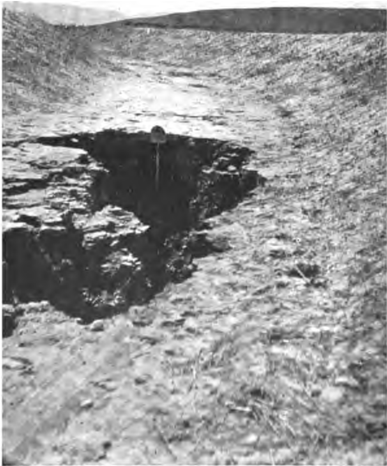
FIG. 73.—Cave Developed in Bottom of Canal, Flathead Indian Reservation.
